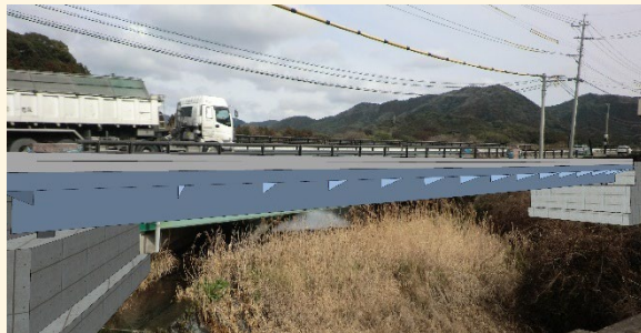
Shin-Asakura Bridge, for which we used green steel for the first time
